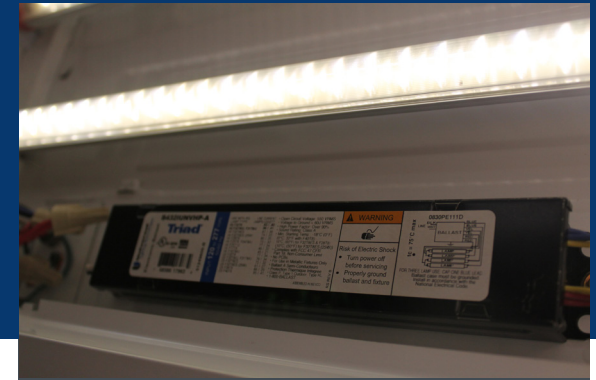
Type A TLED uses the existing ballast. Photo credit Michael Myer, PNNL
