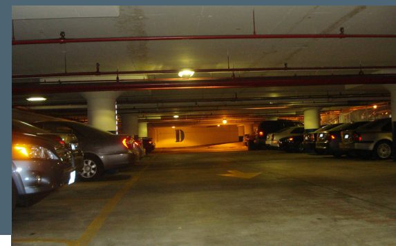
Integral occupancy sensor in parking garage luminaire increases output when motion is detected. Photo credit Akoya, U.S. DOE
