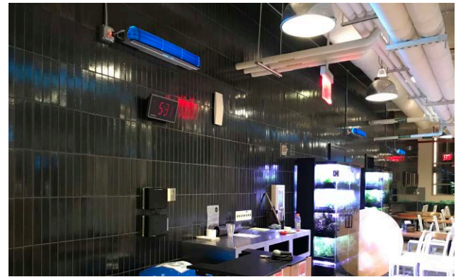
Example of wall-mounted, louvered upper-room GUV luminaires (emitting some blue light) in the field. Photo by PNNL
